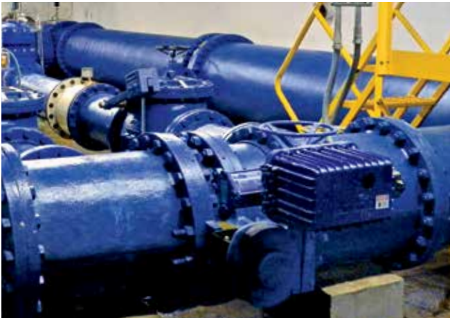
With investment capital from KKR, Bayonne Municipal Utilities Authority has made numerous system upgrades such as replacing deteriorated equipment in the North Arlington gatehouse (above) with modern water mains (below) that handle 8.5 million gallons of water daily.
